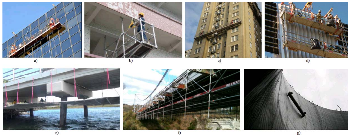
Figure 1. Practical Uses of Suspended Scaffolding Systems (Url-1a-g [1])
