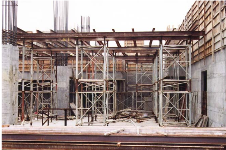
Figure 1. Independent Heavy-duty Scaffolds Assembled on Construction Sites of a High-tech Plant at the Central Taiwan Science Park
