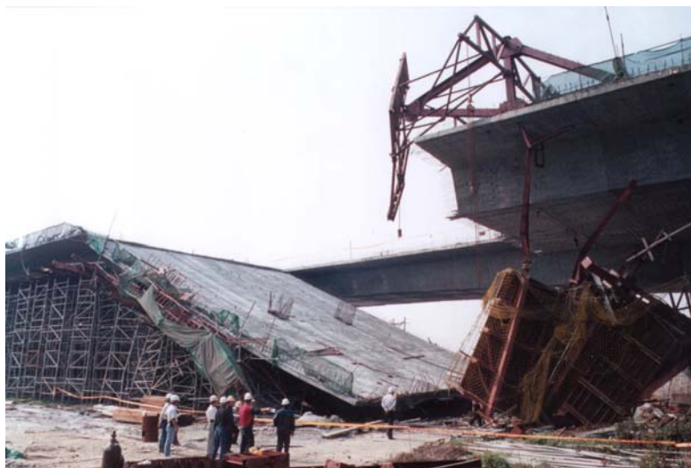
Figure 2. Collapse Scene of Independent Heavy-duty Scaffolds on Construction Sites of a Bridge in Zhunan Section of National Freeway No. 3
