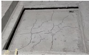
(b) The cracks of composite slab
