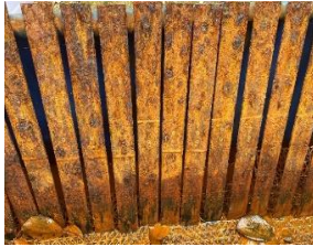
Fig. 1 Specimen corrosion site
