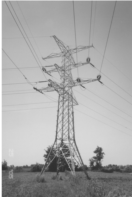
Figure 4. View of Transposition Support with Tension Insulator Sets
