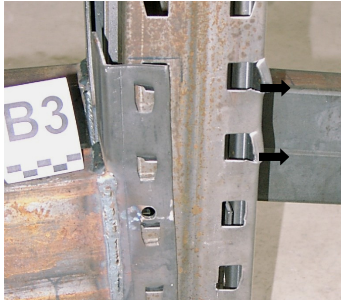
Figure 6. Tearing of the Column Web Observed during the Tests
