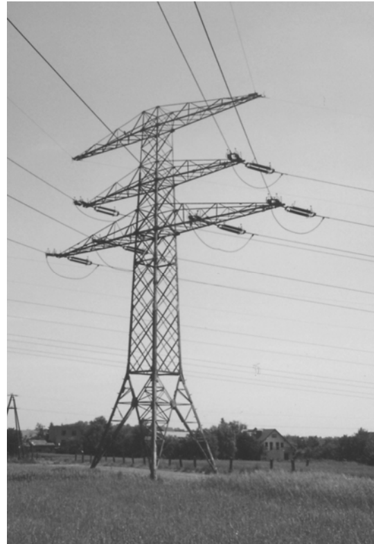
Figure 3. View of Angle Support with Tension Insulator Sets
