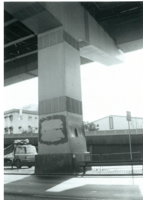
Figure 1. Steel Box Section Bridge Pier Damaged During Hyogoken-nanbu Earthquake Near Kobe City in Japan on January 17, 1995
