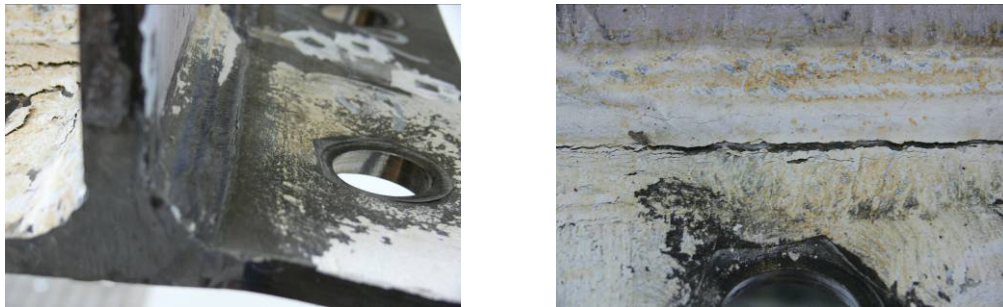
(a) Mode A: Cracking of the End Plate in the Heat Affected Zone (Specimen EEP_10_2(M27))
