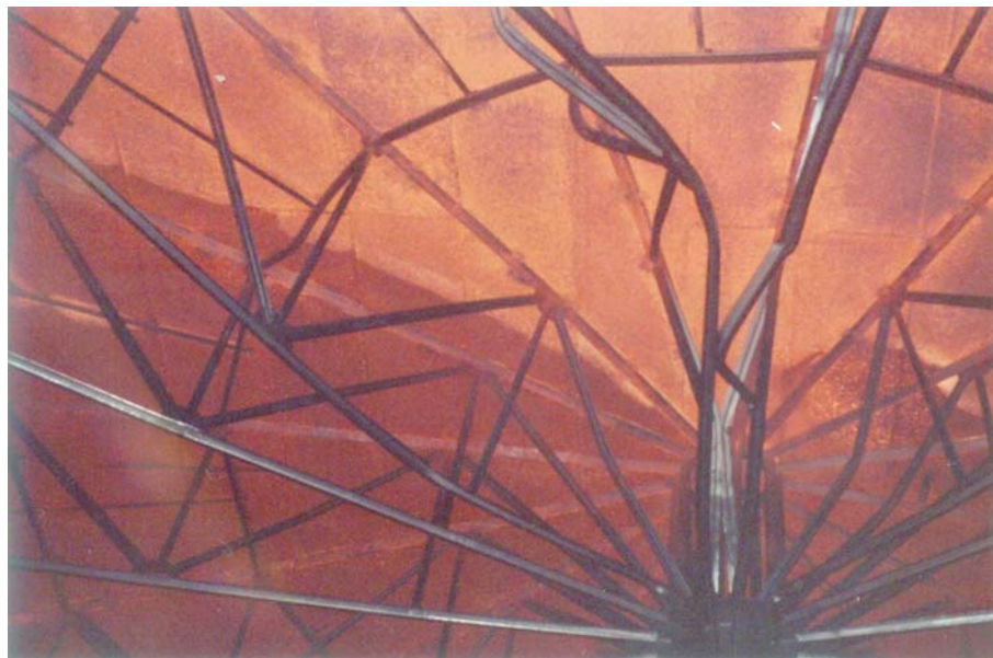
Figure 8. Deformed Roof Trusses in the Vicinity of the Central Column
