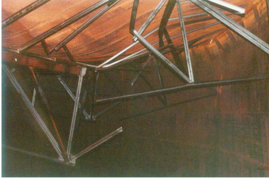
Figure 7. Broken Roof Trusses
