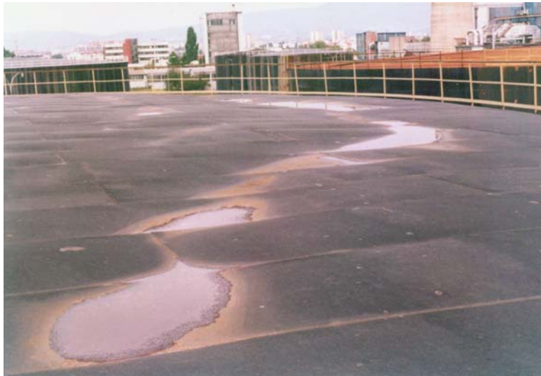
Figure 10. Depressions on the Roof Surface
