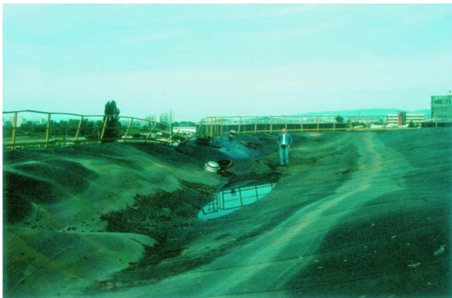
Figure 6. Form of Depression on the Roof Surface
