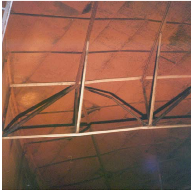
Figure 9. Damaged Roof Truss Members
