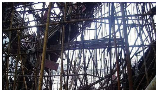
Figure 1. A Collapse Example of STCF using as Shoring Systems
