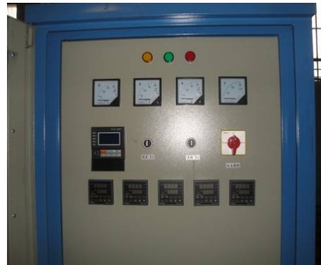
Figure 9. View of Control Box of Heating Furnace
