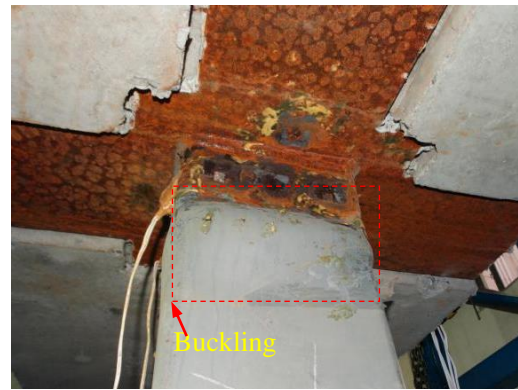
(b) Buckling of steel tube
