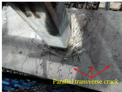
(c) Parallel transverse cracks on the RC slab
