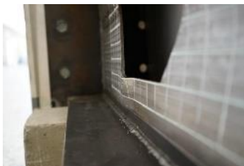
(c) Local buckling of hole angle No. 4
