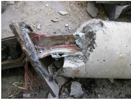
(a) Buckling of unrestrained connection segment and cracked concrete
