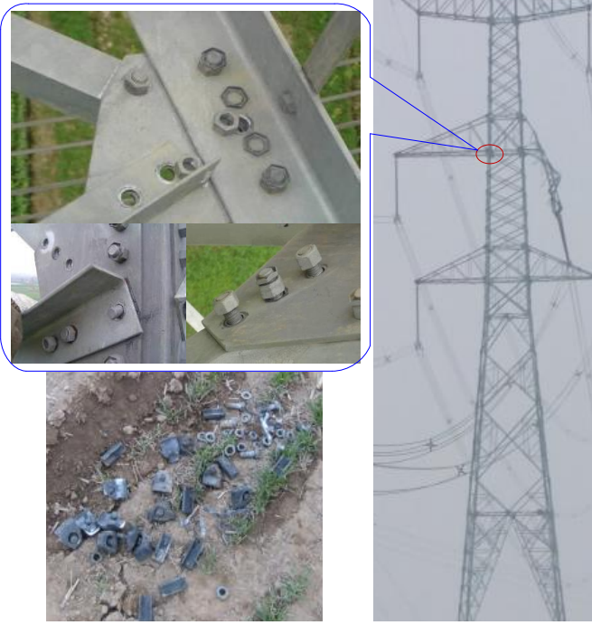
Fig. 2 Tower cross-arm failure accident caused by bolts loosening
