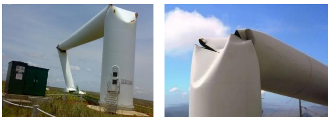
Fig. 1 Steel tower collapse accident caused by instability failure
