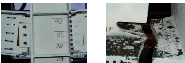
(a) Failure mode of the WUF connection
