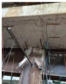
(a) Cracks penetrate between the upper and lower flanges of the slab
