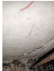
(c) Falling of concrete block of floor slab
