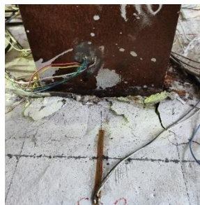
(b) The floor concrete is crushed and hunched up
