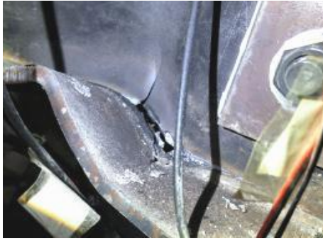
Fig. 12 Beam flange failure
