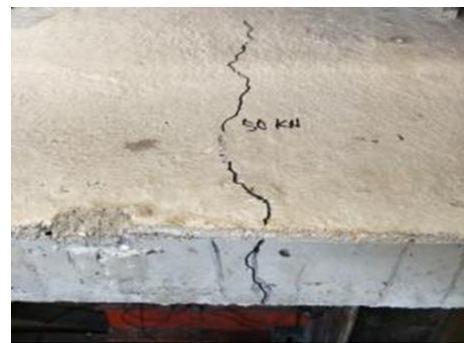
Fig. 10 Crack on the concrete floor
