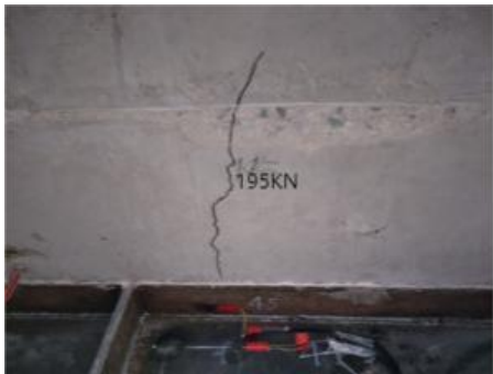
Fig. 7 Crack on the concrete floor
