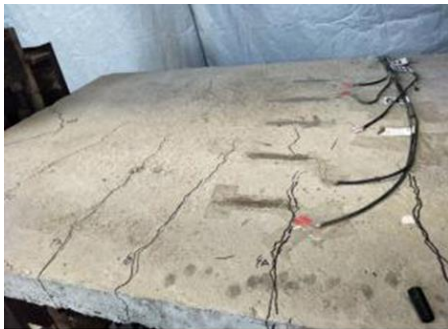
Fig. 8 Crack on the concrete floor
