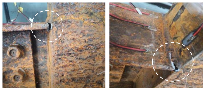
(c) Local damage
