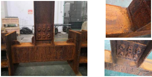
Fig. 5 LZ-2 appearance after corrosion
