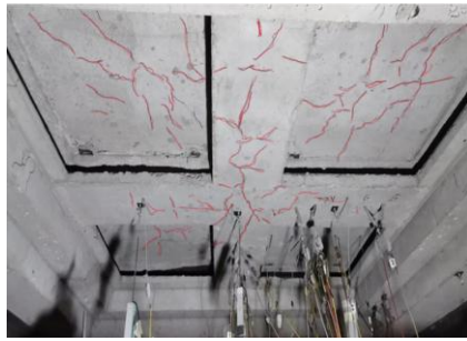
(b) Cracks and failure in test
