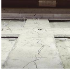
(a) The cracks of ribbed beam
